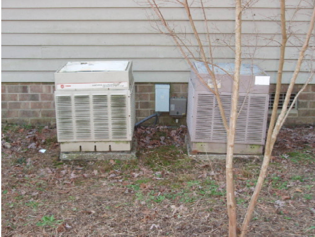
HVAC compressor units
