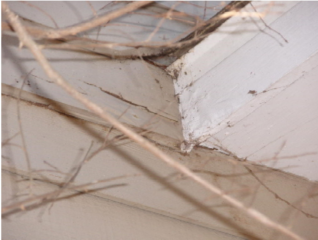
Exterior moisture damage near garage
