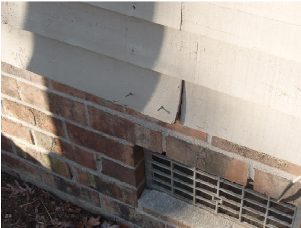
Exterior loose boards
