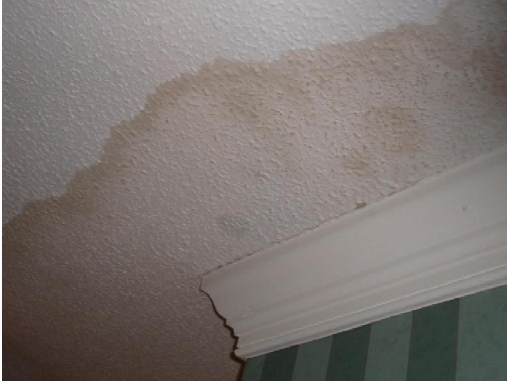
Bathroom stains at 1/2 bath ceiling
