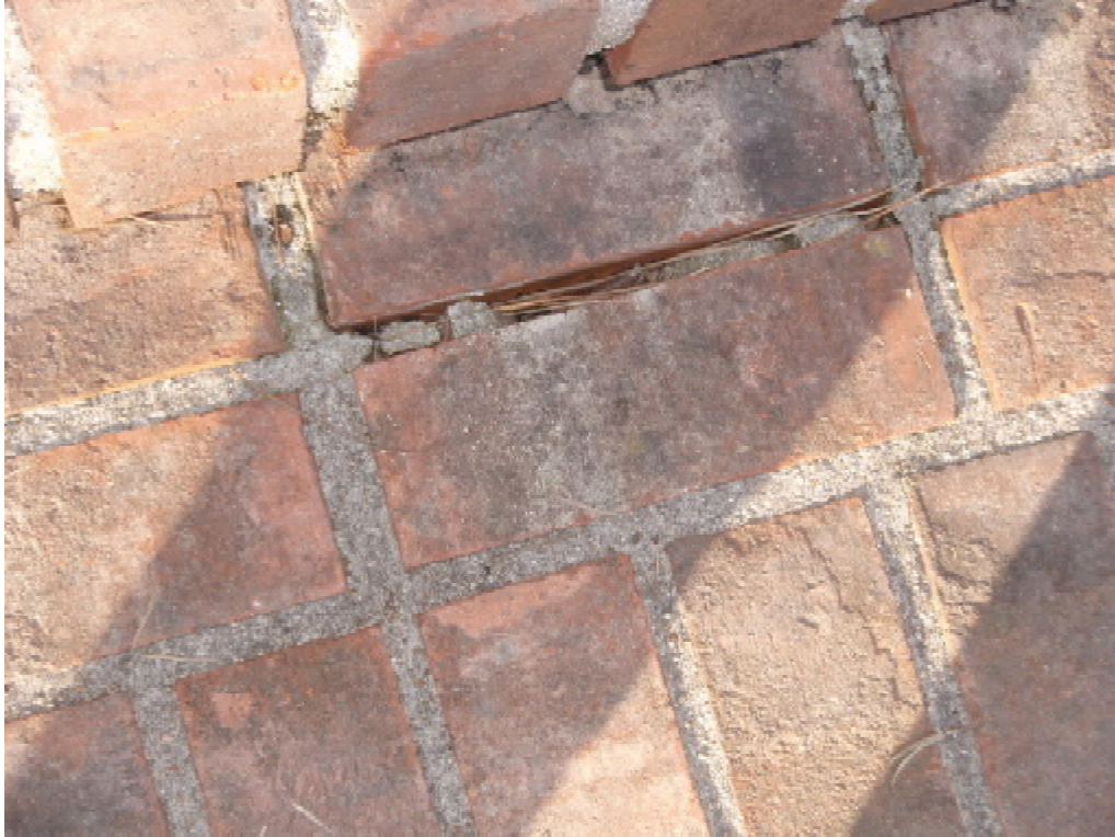
Grounds & Drainage cracks & gaps at front steps
